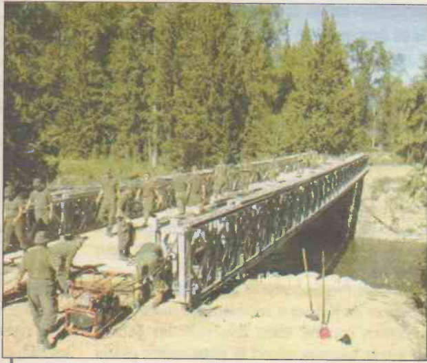
Engineers are hard at work on the Creston Valley, B.C., Bailey Bridge constructed by 44 Field Engineer Squadron. The project was named the Izzy Bridge in memory of MCpl Mark Isfeld, a military engineer killed by a land mine while serving in Croatia in 1994.
