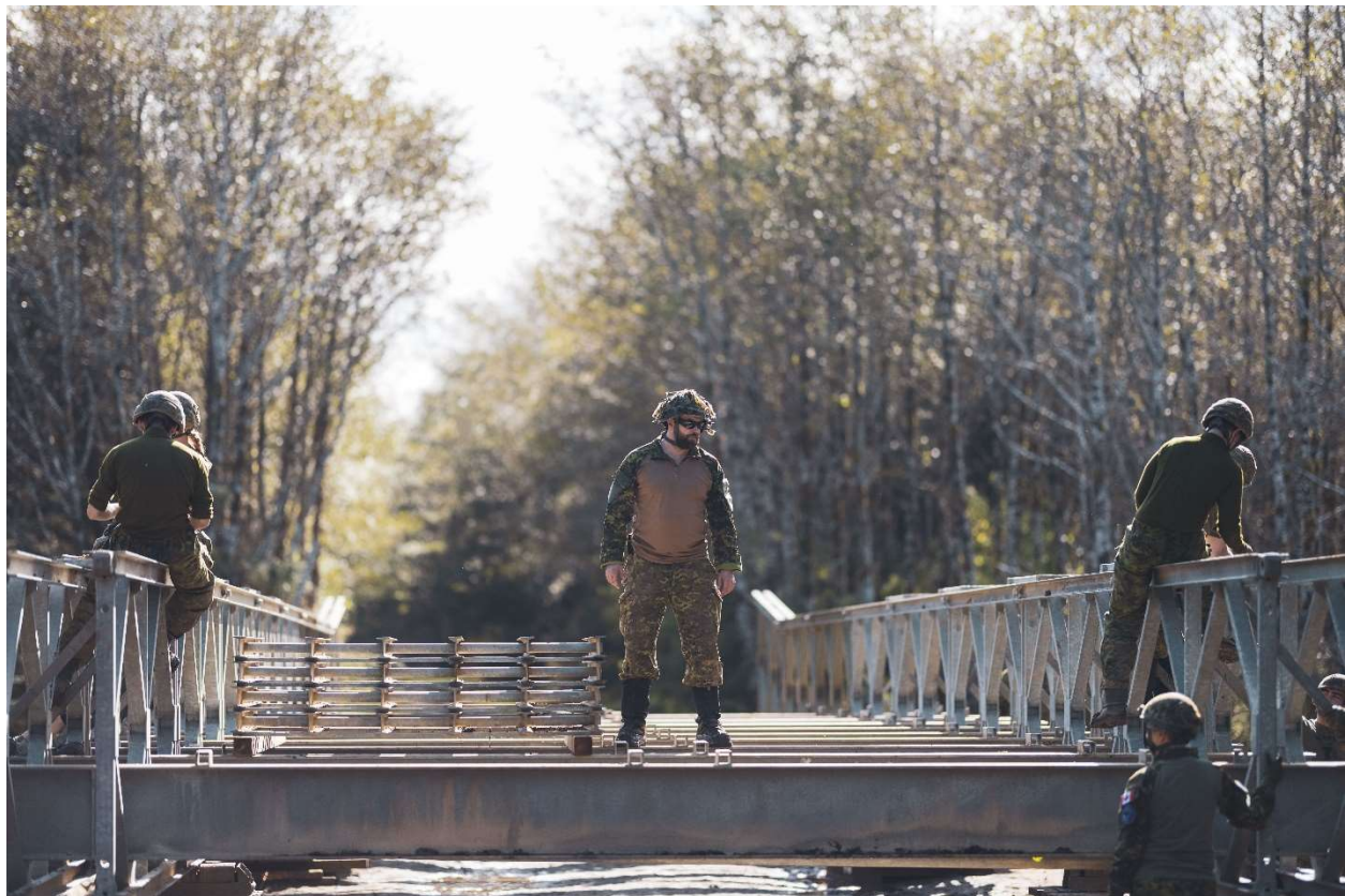
Ex HS 21 – Photo 1: Master Corporal Grasby, from 39 Combat Engineer Regiment, Bridge Commander of the ACROW bridge build, where members of 39 Combat Engineer Regiment built a permanent ACROW bridge for Canadian Forces Detachment Masset, on Ex HAIDA SAPPER, in Masset British Columbia. 25 September 2021. Photo: Private Daniel Pereira, 39 CBG Public Affairs
