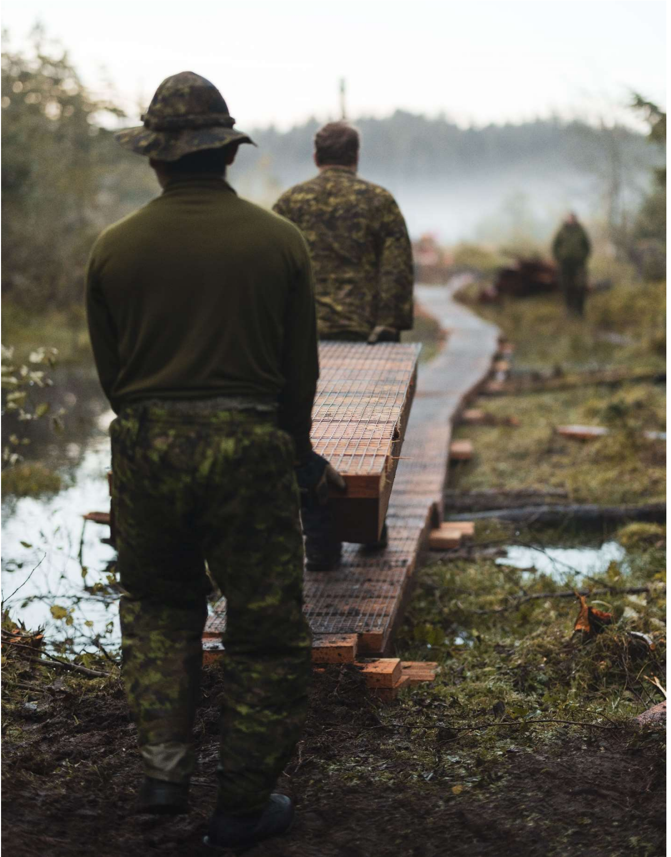
Ex HS 21 – Photo 2: Members of 39 Combat Engineer Regiment construct a boardwalk through a swamp for Canadian Forces Detachment Masset, during Ex HAIDA SAPPER, in Masset British Columbia. 25 September 2021. Photo: Private Daniel Pereira, 39 CBG Public Affairs
